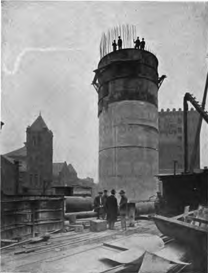
PLATE 231.—Contract 66. Shaft 23. Concrete Caisson which was Sunk to 100 Feet below Ground-water under Maximum Air Pressure of 45 Pounds. Length of Caisson 123 Feet. Sunk to ground-water level and built to maximum height before putting on air pressure.
